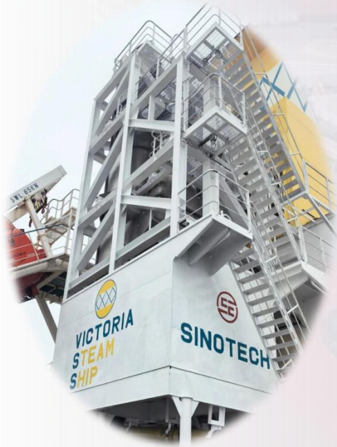
EGCS (Exhaust Gas Cleaning System)
